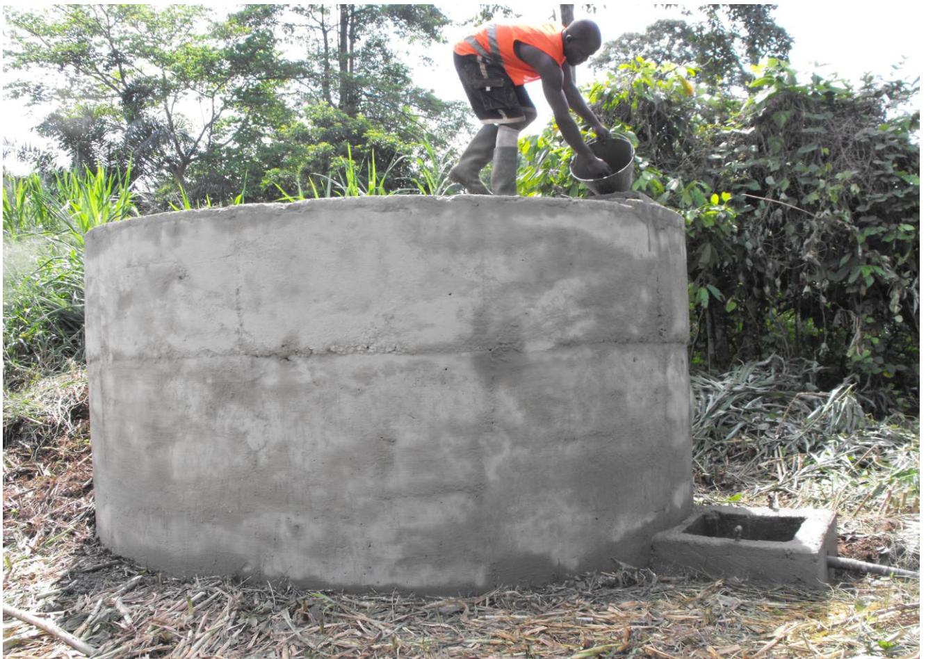
Wassertank in Ebonji
